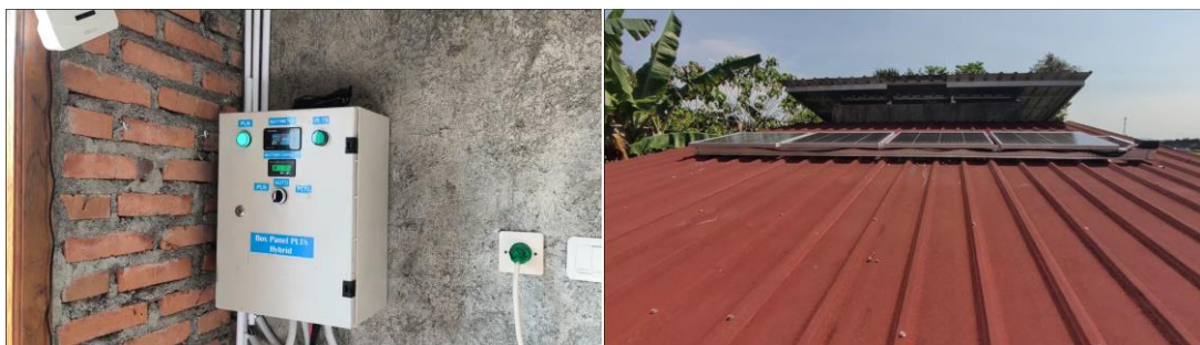
(a) (b) Figure 9 PV Systems, (a) Control Box, (b) PV Panels
