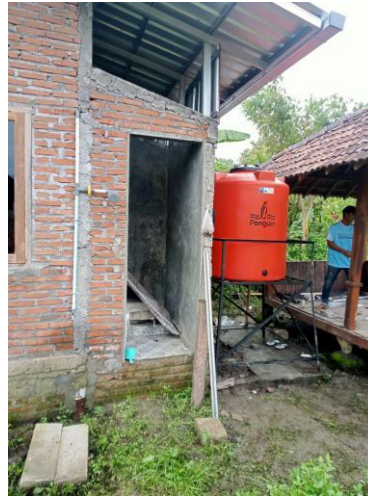
Figure 10 rainwater harvesting system
