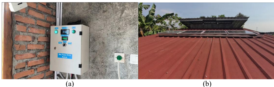
Figure 9 PV Systems, (a) Control Box, (b) PV Panels
