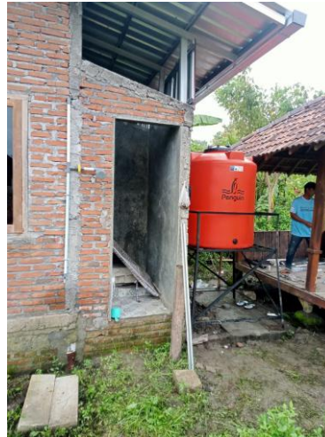
Figure 10 Rainwater Harvesting System
